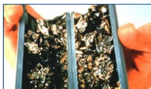
Water intake pipe blocked by zebra mussels
